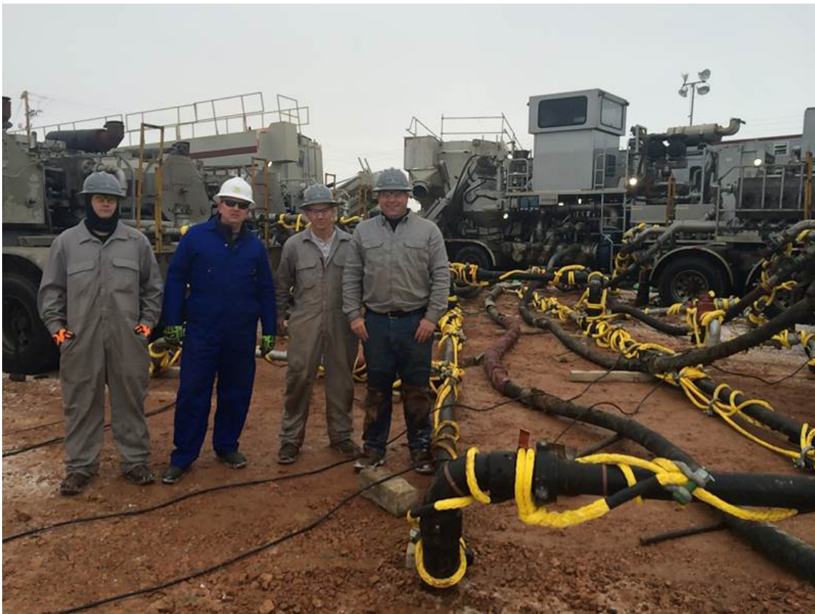
Bruce Hartin (in blue) and representatives of Crown Supply, Inc. on a recent large-scale Gangline™ installation in the Bakken Shale in North Dakota.
